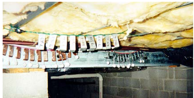
Figure 5 - Stud Specimen in Leonardtown Site Crawlspace
